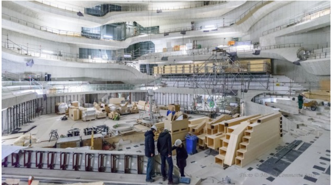
The construction of the great hall. A special wall cladding system, the so-called "white skin" will provide for good acoustics
