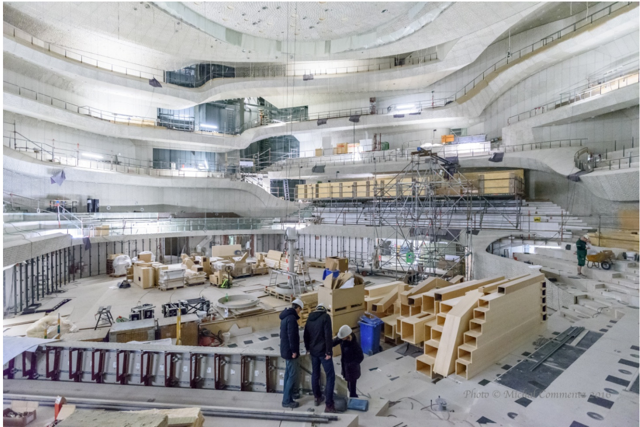
Interior view of Elbphilharmonie's Great Concert Hall under construction (Image: M. Commentz)
